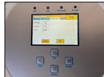
Figure 3: Battery Shut Down settings
