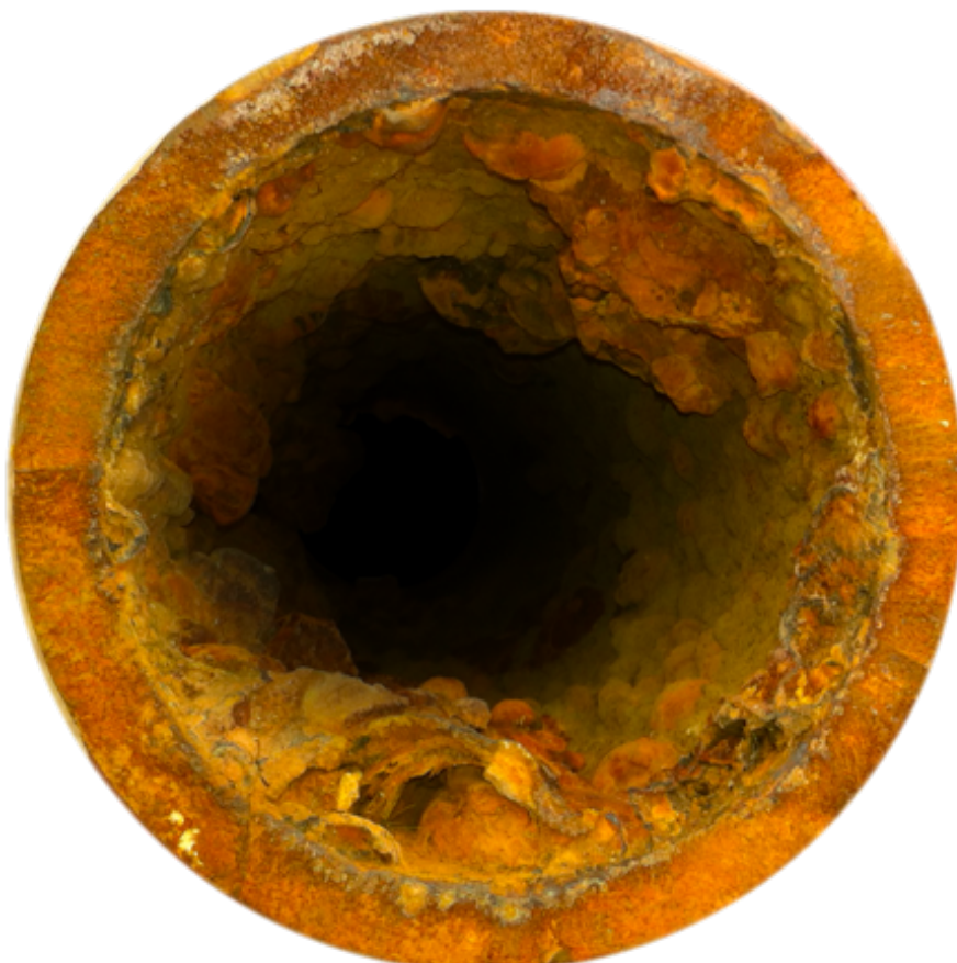
Corrosion and rust
